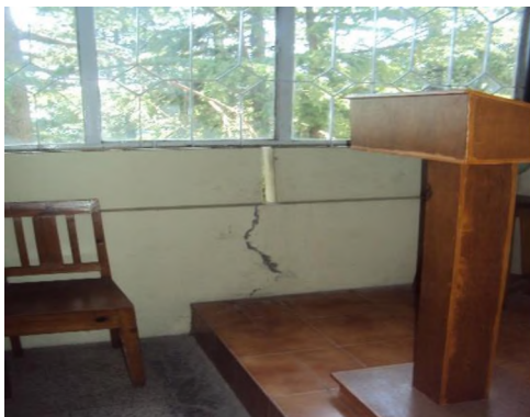
Fig. Wall Cracks
