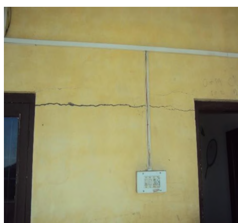
Fig. Wall Cracks
