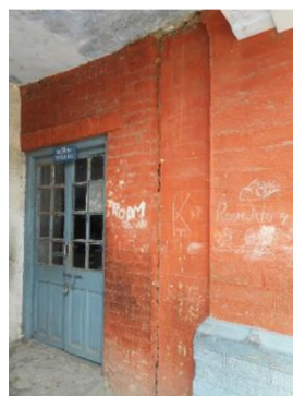
Fig.: Joint Crack
