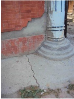
Fig.: Foundation Crack
