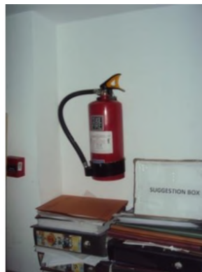
Fig.: Fire Extinguisher
