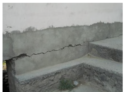
Fig.: Foundation Crack
