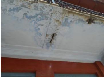
Fig.: Reinforcement Corrosion
