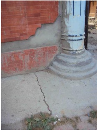
Fig.: Foundation Crack
