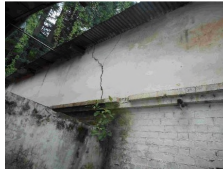
Fig.: Outside Wall Cracks
