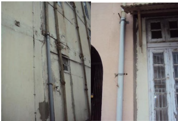
(Fine Cracks) Fig.: 9 {ii (moderate cracks)}
