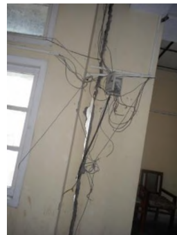
Fig.: Joint Crack (i)
