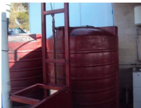
Fig.: Water Tank
