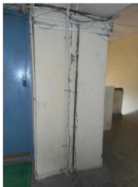
Fig.: Joint Crack (i)
