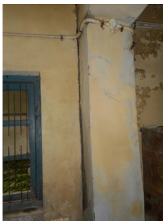
Fig.: Joint Crack (iii)
