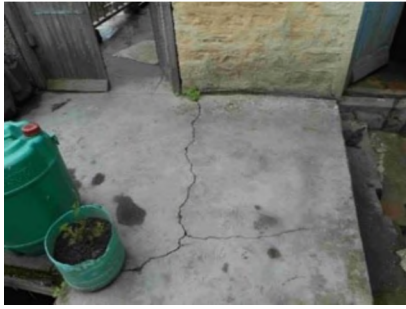
Fig.: Foundation Settlement
