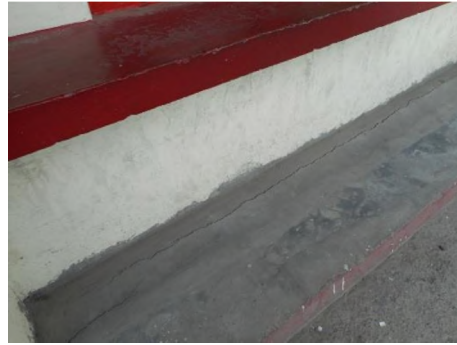
Fig.: Foundation Crack
