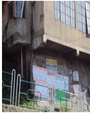
Fig. : Reinforcement corrosion
