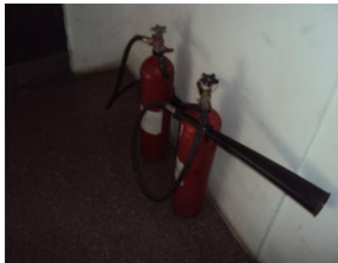
Fig.: Fire Extinguisher
